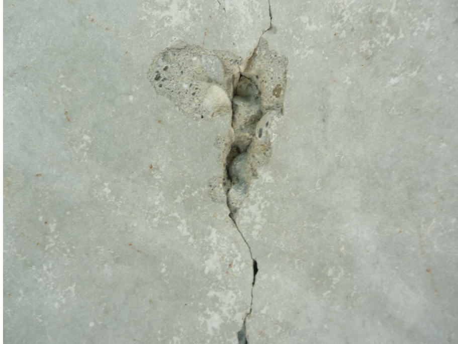
Figure 2. Spalling at NE crack location
