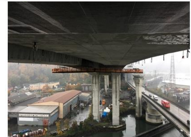
Temporary work platforms enable crews to do important stabilization work on the West Seattle High-Rise Bridge, and offer a unique view of the Low Bridge.
