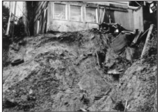
DPD staff inspected nearly 400 private properties in Seattle for landslide damage after the 1997 New Year's Day storm.
